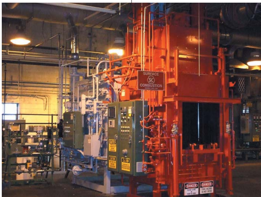
Retrofitted Surface Combustion Allcase furnace at Metal Improvement for running FNC process.
